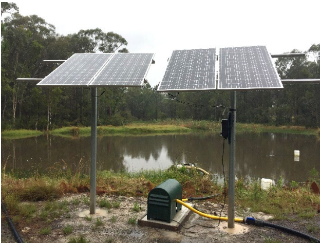
Figure 7: Solar-powered pump station and a single suction line managed by Barung Landcare Association next to the dam in the south section of Brannocks Environment Reserve.
