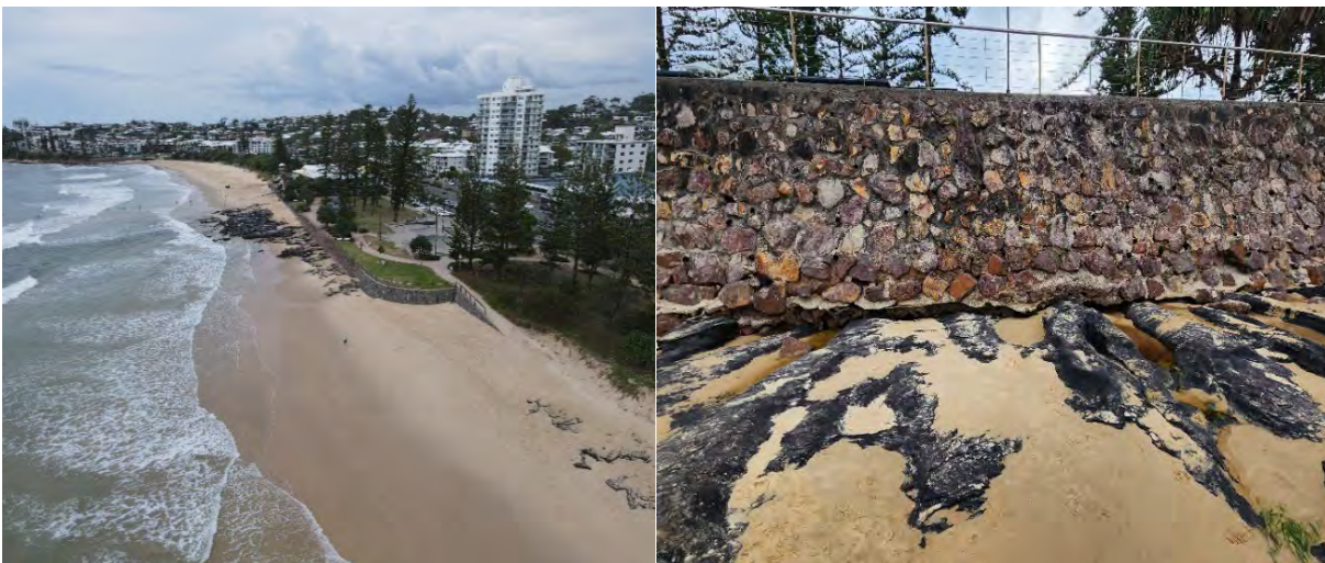
Figure 14-2: Northern seawall at Alexandra Headland Beach. Left: Skatepark and SLSC looking south. Right: Scouring underneath the seawall (JBP 2023)
