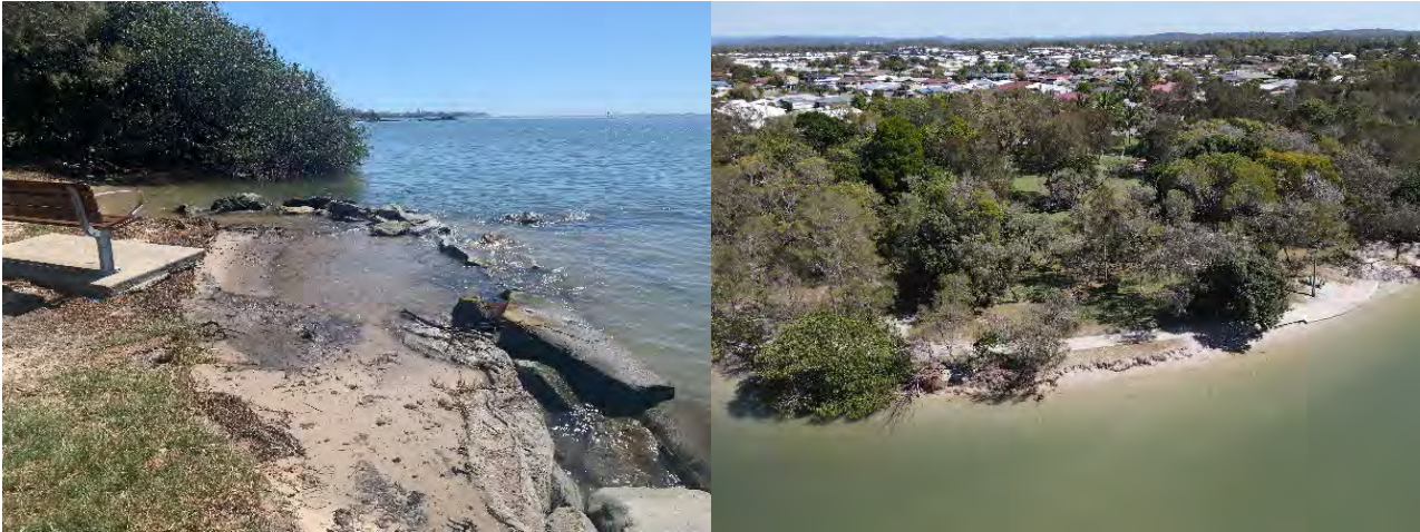
Figure 39-2: Estuary Unit E7. Left: Overtopping and scouring of revetment near Roy Street. Right: Erosion along the shoreline at Bells Creek entrance (JBP 2023)
