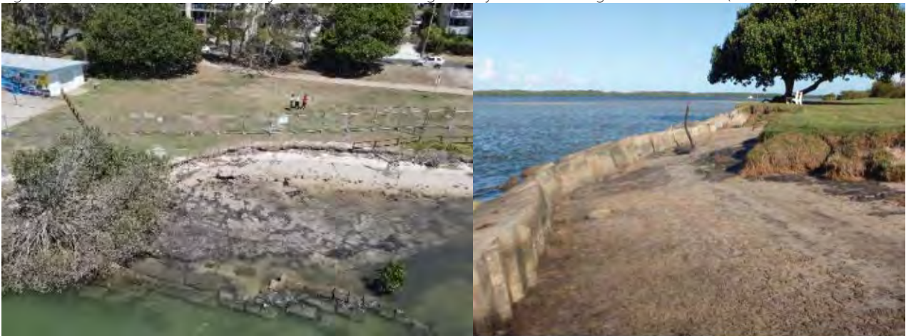
Figure 37-3: Left: Erosion at the failed seawall (JBP 2023). Right: Images of concrete blocks from previous SEMP 8
