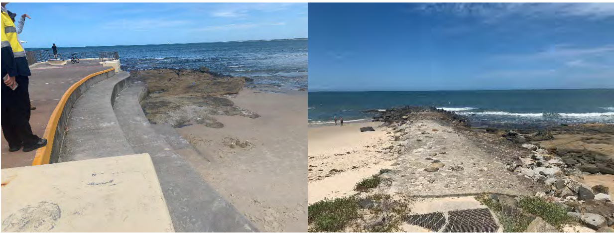
Figure 33-3: Left: General condition of the terraced seawall. Right: General condition of the groyne (JBP 2023)
