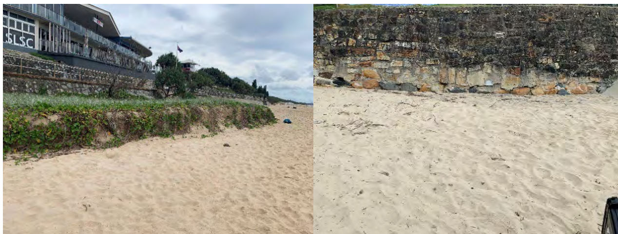
Figure 4-2: Left: Transition beach and dune towards the south of the unit. Right: General condition of the wall showing minor loss of mortar (JBP 2023)
