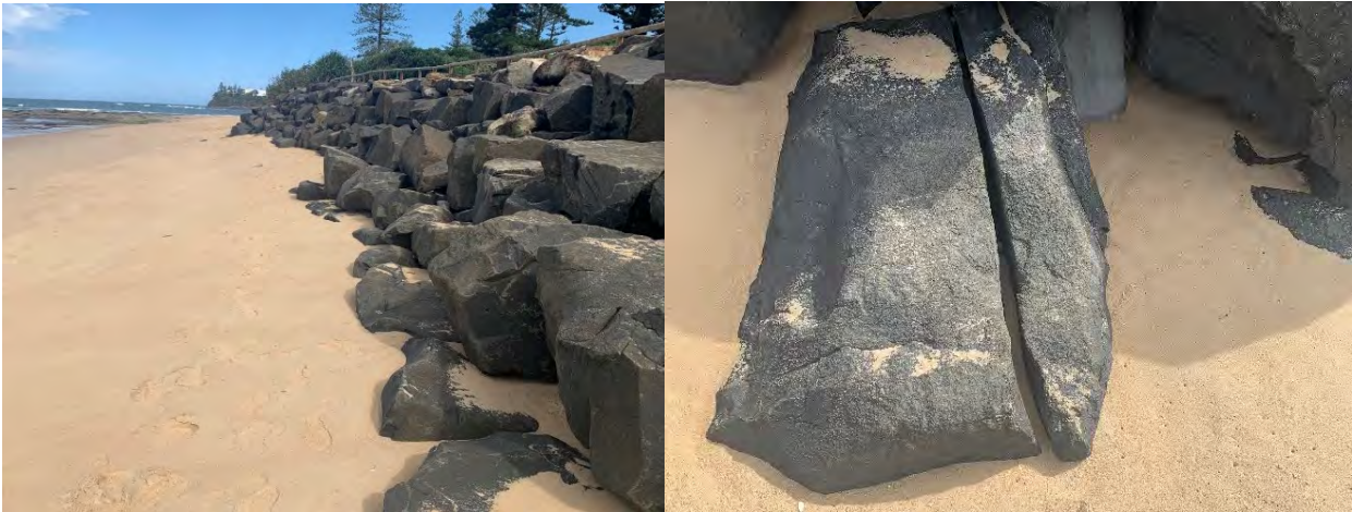
Figure 26-2: Left: Dicky Beach protection structure looking south. Right: Spalling rock (JBP 2023)
